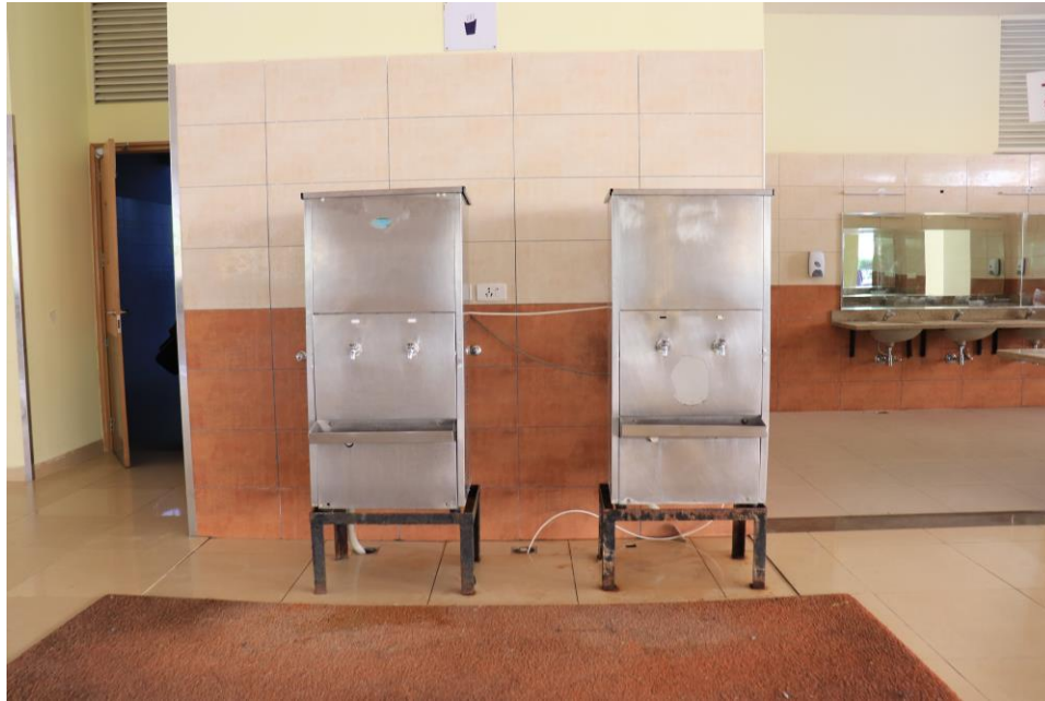
Picture 5: Water Station installed in the food mess
